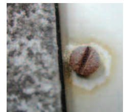
Non-stainless steel fasteners in stainless steel panels suffer accelerated and severe corrosion.
